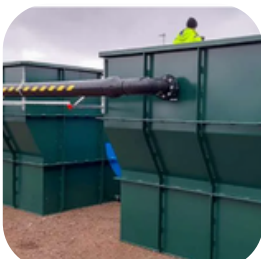
MBBR reactor: Moving bed reactor utilizing aerobic bacteria.
